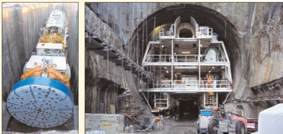
Figure 2.4.1 TBM is seen at the start position and while disappearing on its route.
